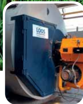
Gas Fired Steam Boiler
