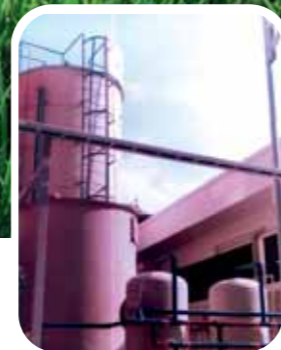
Sewage Treatment Plant
